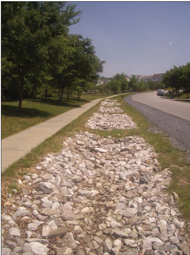
This swale can capture runoff from the adjacent road. Some swales, like this one, are lined with rocks, while others are lined with vegetation and other media like mulches.
