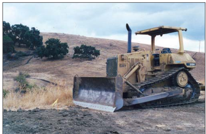
Temporary Best Management Practices can help limit damage to vegetation and soils during construction.
